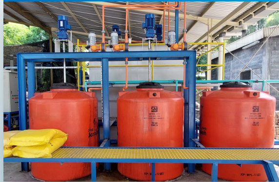
UNIT CHEMICAL DOSING
