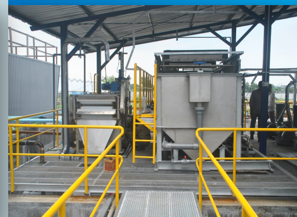
WASTE WATER TREATMENT SYSTEM
