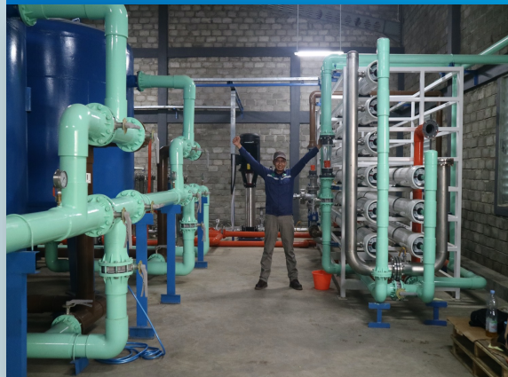
WATER TREATMENT SYSTEM
