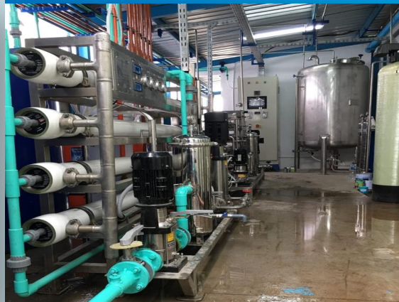
PURIFIED WATER SYSTEM
